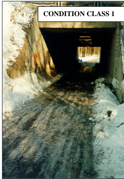
Figure 12. A problematical pedestrian and cyclist underpass
