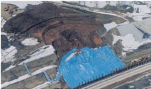
Figure 2 Slope failure site (Under construction)
