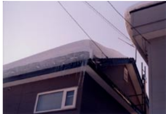
Figure 17 Melting rooftop snow
