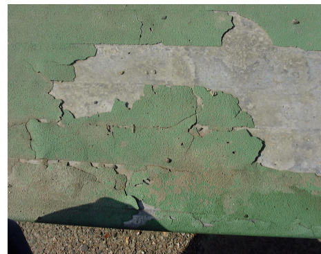
Figure 3-3 Polyurethane (thin film) Peeling
