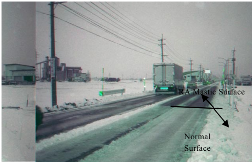
Figure 7.4 Pavement Surface Condition of RA Mastic in Winter
