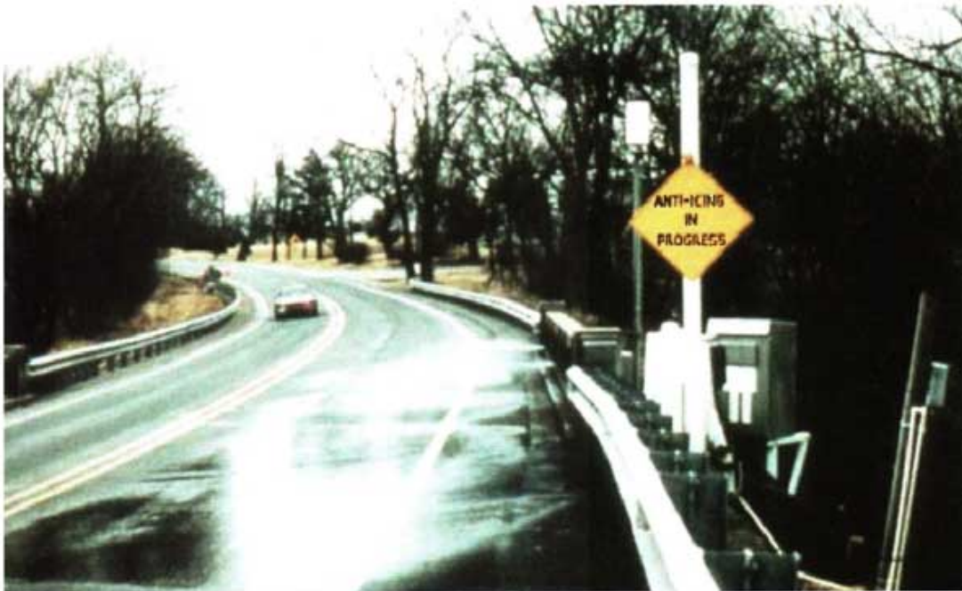
Fixed overpass anti-icing spray installation. Photo courtesy of CRYOTECH Deicing Technology
