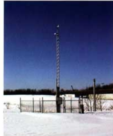
Typical RWIS installation
